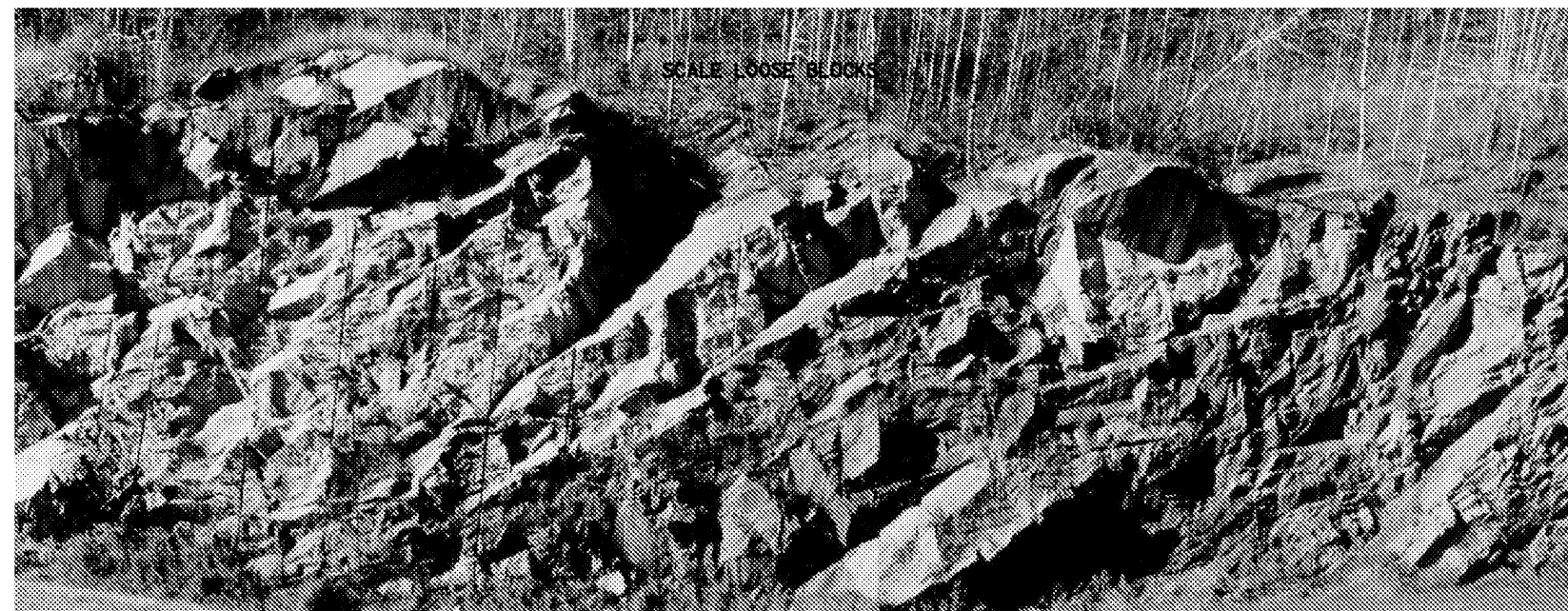
APPROXIMATE MM 71.18 SCALE LOOSE BLOCKS ON CREST
